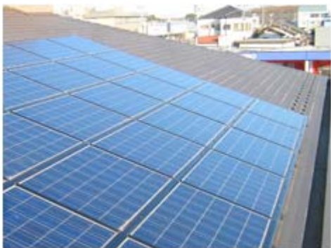
Rooftop solar panels
