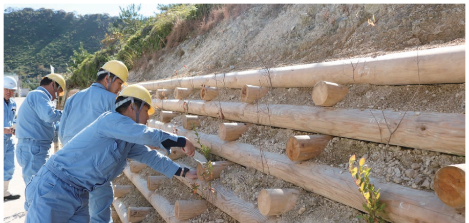
Using logs from windfall trees to retain soil and then planting trees in between the logs to further solidify the soil.
