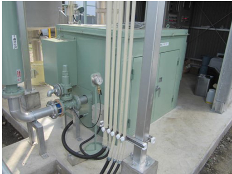
Biological processing facility (aeration blower)
