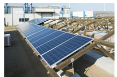
Solar panels and environmentally friendly wooden frames
