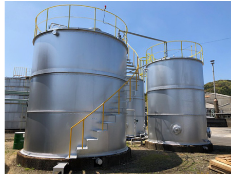
Biological processing facility (aeration tank)
