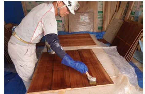
Cleaning drainage water stains
