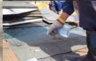
Water is sprayed over asbestos materials to prevent the dispersal of asbestos dust
