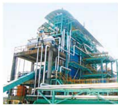
Wood biomass power generation facility which began operation in March 2008
