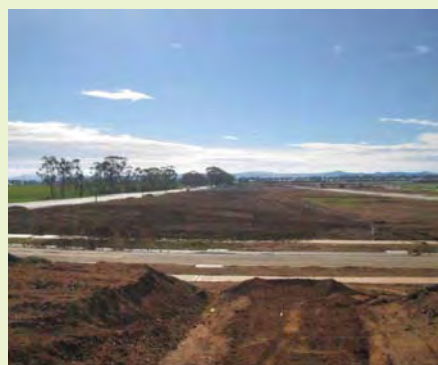
The site in Melton, Victoria where spec homes are scheduled for construction. Sumitomo Forestry subsidiary Alpine MDF Industries Pty Ltd. is also located in the state of Victoria, and will supply MDF (Medium Density Fiberboard) for the project.
